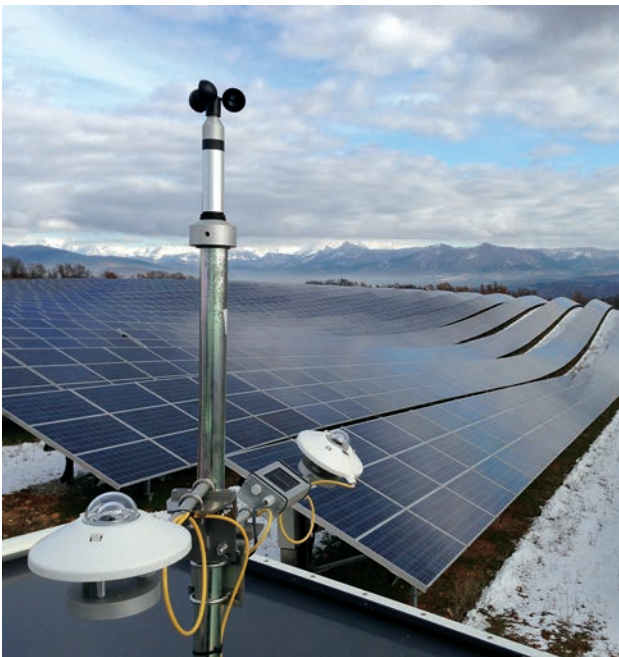
CMP10 pyranometers measuring horizontal and tilted global radiation
